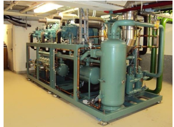
Figure 1: Compressors of refrigerant plant
